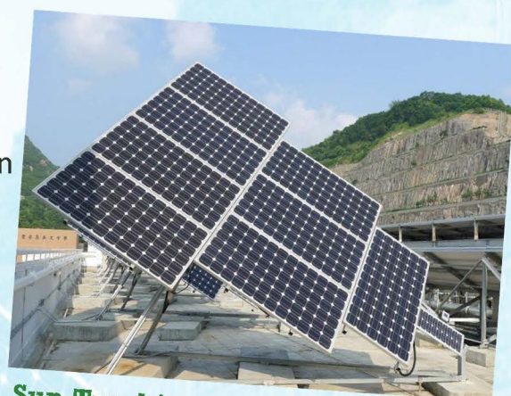
Sun-Tracking Photovoltaic Panels
